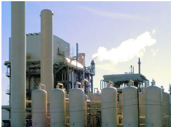
Figure 16: Typical reformer plant; The Linde Group
