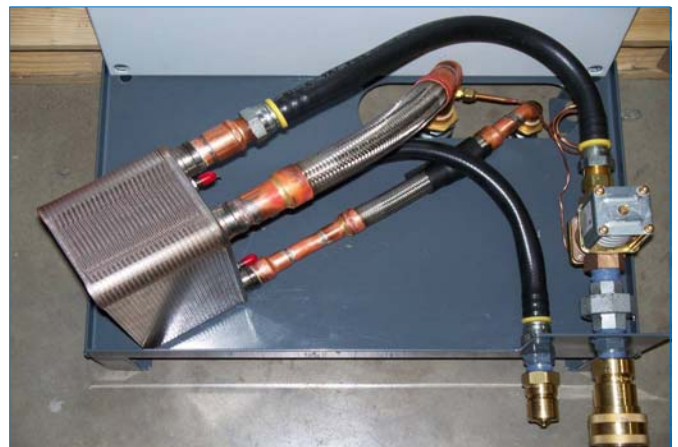
Figure 6. Liquid-to-liquid condenser module installed in demonstrator system with additional sensors and metering components.
